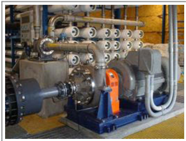
SSD-500 with HPB-500 SWRO Facility
