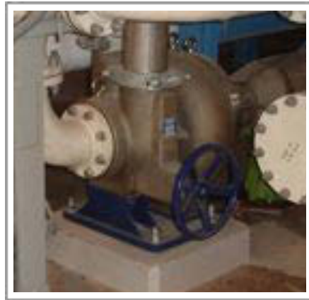
HPB-1000 in Jeddah, Saudi Arabia
